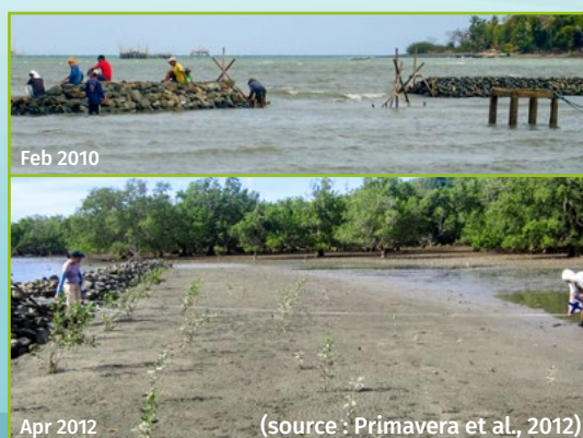
Figure 6 Example of the installation of breakwaters to promote the recolonisation of a mangrove forest.
